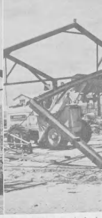
TRABAO RAPIDO a worde haci k building's steel frame. Steel cables were merely secured to staa di oficina Zone 2. Cable di staa biganan y nan un poten
